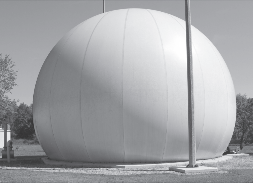
Biogas reservoir in Zdroje Sewage Treatment Plant. Photo by Łukasz Wyka
